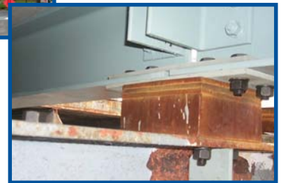
Steel bolstered connections to longitudinal stringers were designed to make new deck surface match the existing surface.
