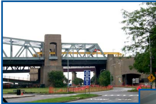
PCSCD units were installed on the through trusses of the Bronx Approach to the Triborough Bridge in New York City, NY.
