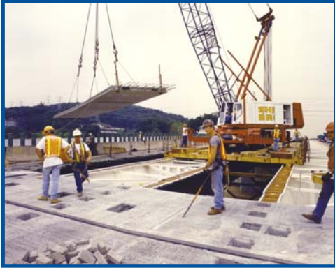
Crowned transverse deck panels were set at the rate of over 15 per day.
