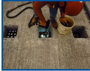
Shear studs were welded to the beam flanges after longitudinal post tensioning was complete.
