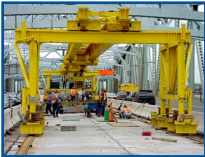
A special erection crane, designed by the Perini Corporation, was used to erect the panels.
