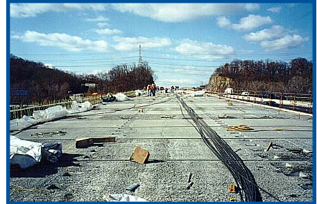
Deck panels were post tensioned longitudinally from one end of the bridge to the other end.
