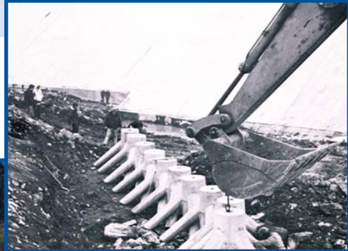
Sta-Pod™ Concrete Armor System for energy dissipation and toe line stability at Jamesville Dam rehabilitation Project.
