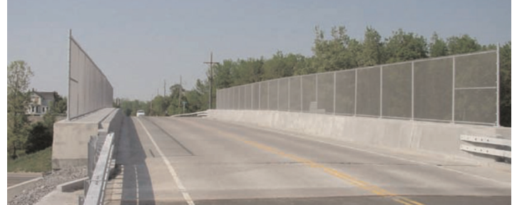
Safety barrier protects edge beams on the Hook Road Bridge in Rochester, NY
