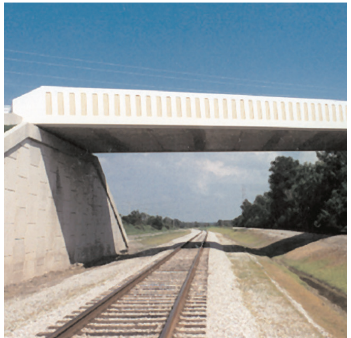
Safety barrier protects edge beams on the Hook Road Bridge in Rochester, NY.
