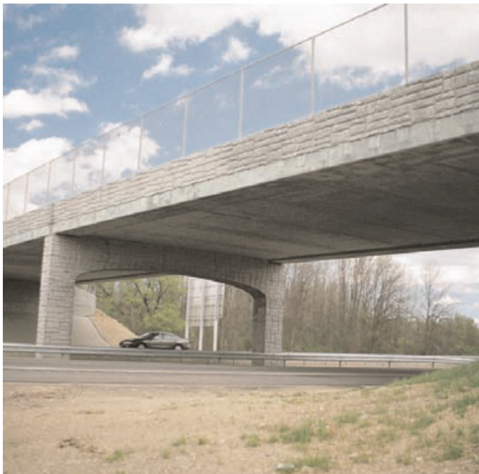
Hook Road over The New York State Thruway, Rochester, NY. Form liner finish on edge girders matches abutments and the pier.
