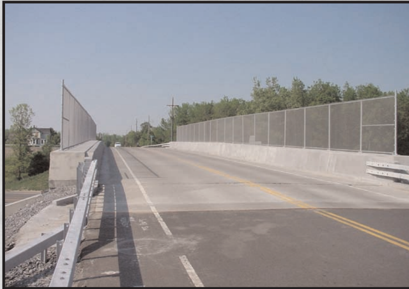
Safety barrier protects edge beams on the Hook Road Bridge in Rochester, NY.
